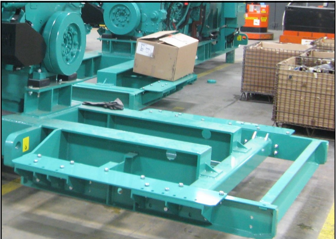
FIGURE 44. COMPLETED INSTALLATION OF THE SKID WING PLATE ASSEMBLY
